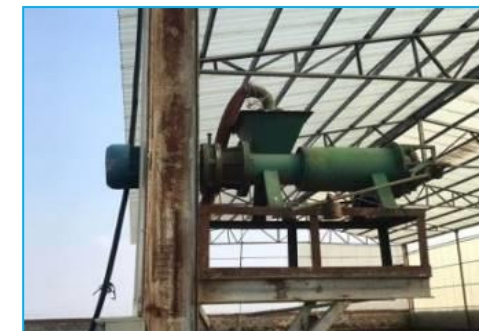
c) Sewage disposal through cow manure drain trap
