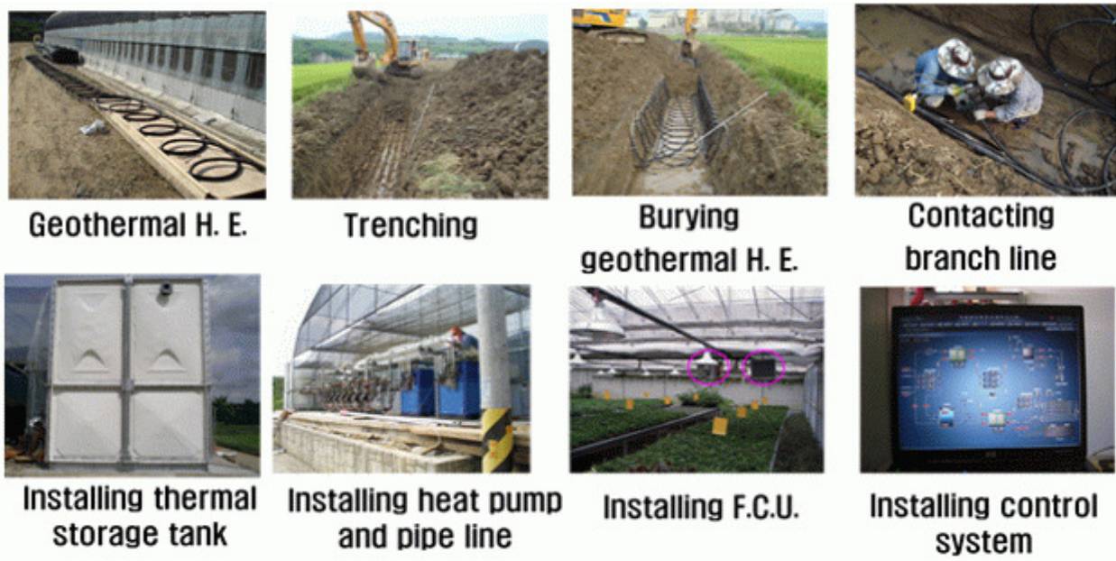
Fig. 12 Vertical-typed geothermal heat pump system for greenhouse heating
