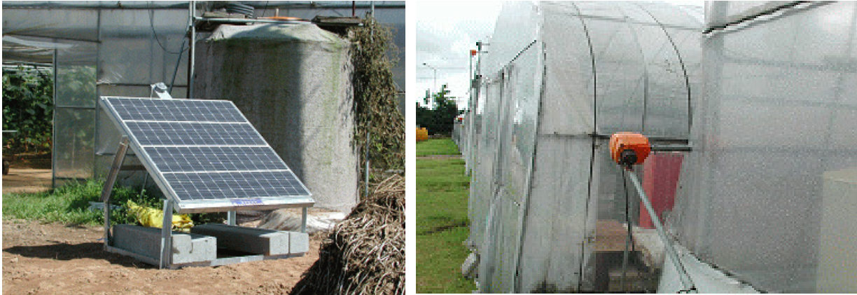
Fig. 13 Greenhouse window opening using the solar PV system
