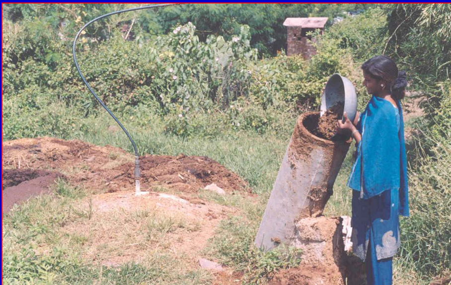
Janta Biogas Plant
