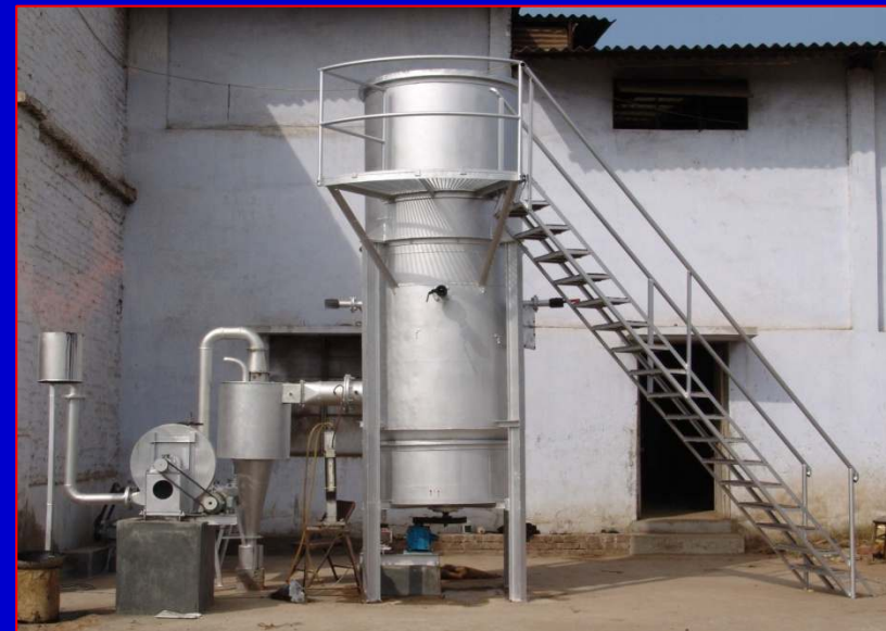
Biogas plant for chicory
