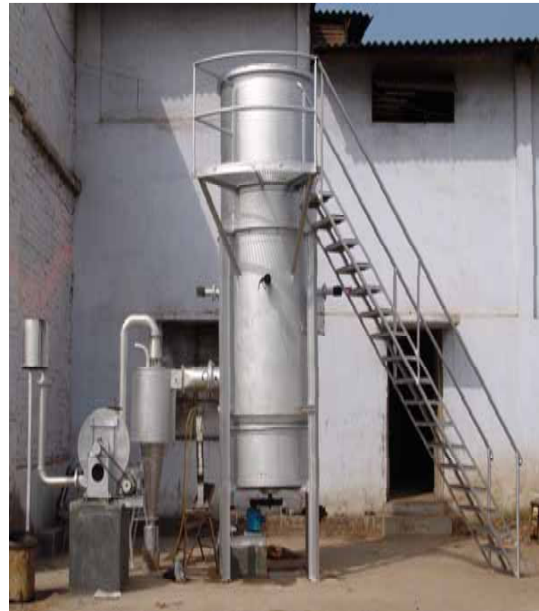
Producer gas system installed in an industry near Anand (Gujarat) for chicory roasting
