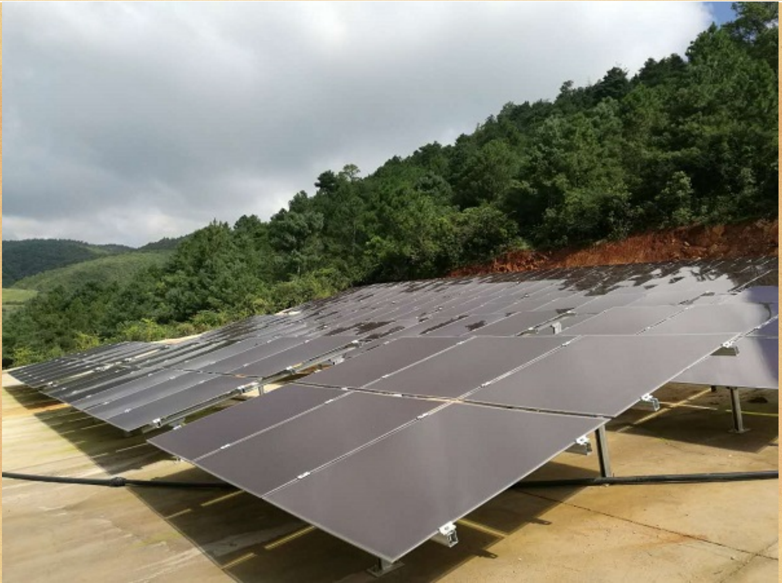
Tian chong qing Solar pumping station
