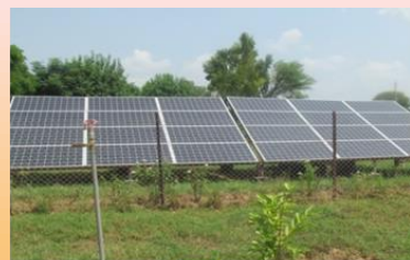
PV Modules for Solar Energy
