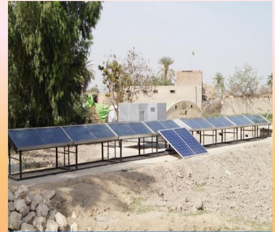
Solar-Cum-Gas Fired Dates Dryer
