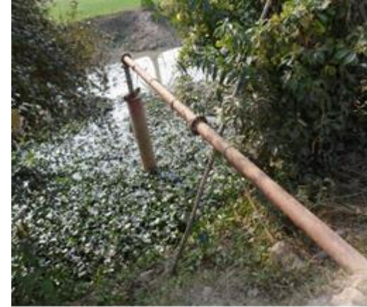
Solar panels are used for powering motors for lifting irrigation water
